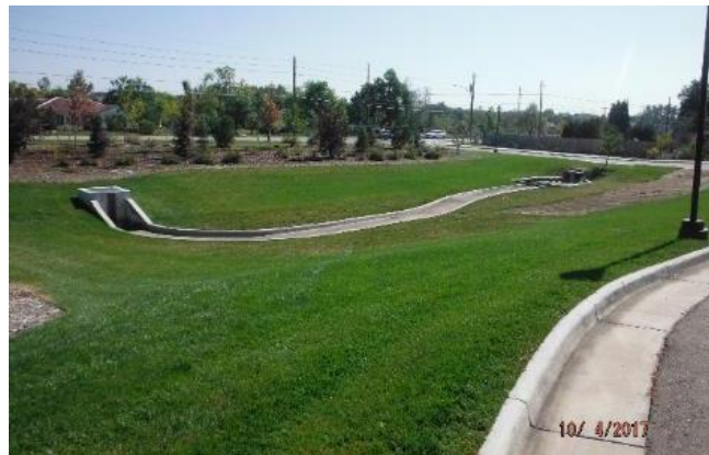
Photograph 5-A. This EDB includes a concrete trickle channel and a micropool with a concrete bottom.
