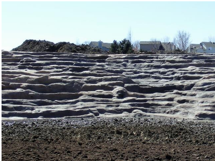
Sculpted Concrete Drop Structure on Airport Creek West of Sheridan Blvd.
