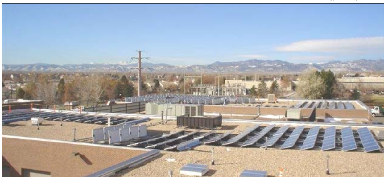
Photovoltaic system (PV) installed on Municipal Services Complex in 2009-2010.
