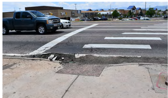
Damaged crosswalk and sidewalk
