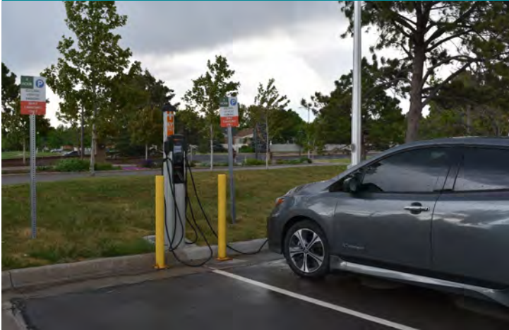
Electric vehicle charging at Westminster City Hall
