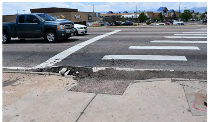
Damaged crosswalk and sidewalk
