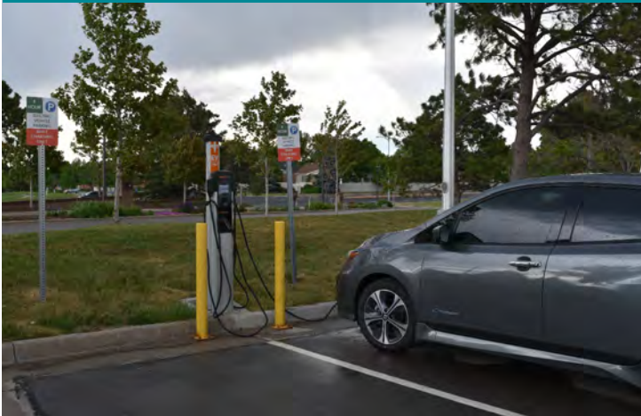
Electric vehicle charging at Westminster City Hall
